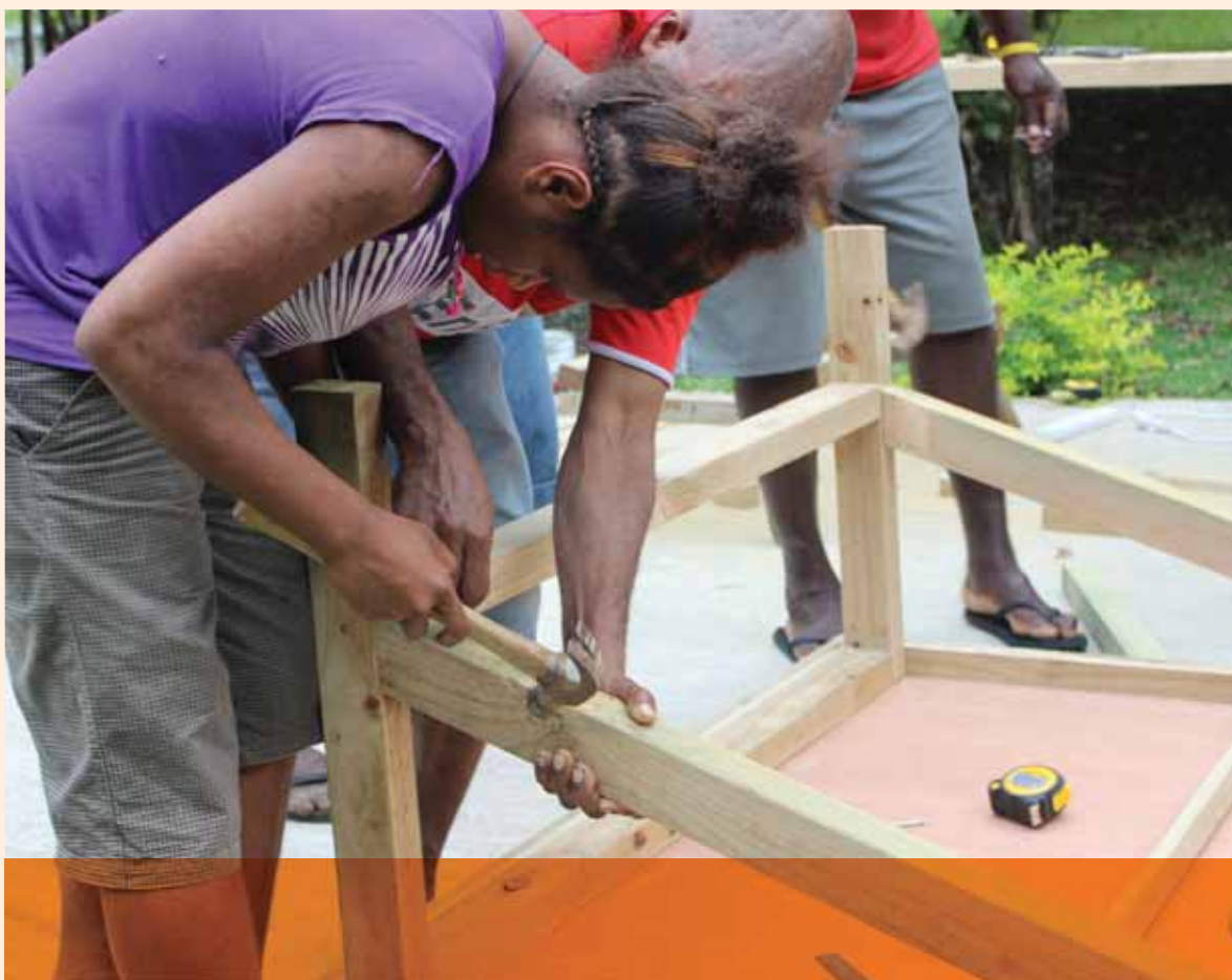
Workshop on building and maintaining food processing solar dryer units, Espiritu Santo, Sanma Province.
