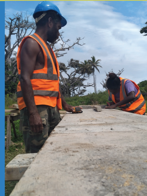
Two construction skills trainees from Namas Lume Vocational Training Centre learning new skills during the construction of the Provincial Area Administration Office on site at Imlao village, South West Tanna.
