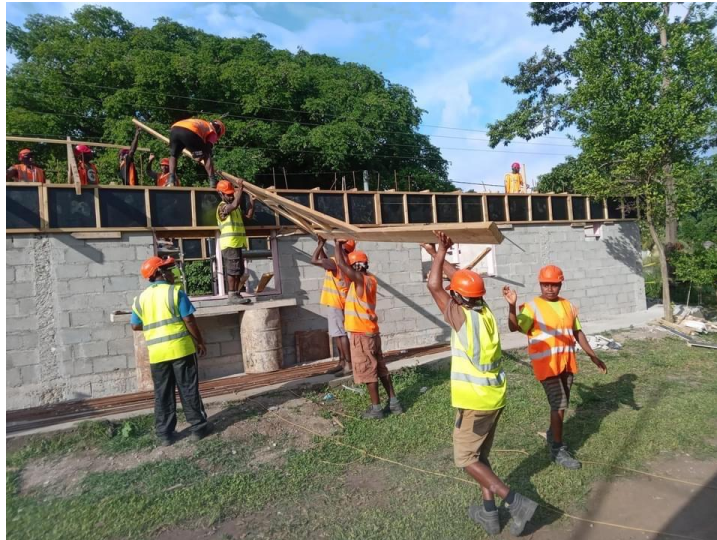
Figure 3: Construction trainees working on the roof of the new Tafea Handicraft Centre in Lenakel, Tanna.
