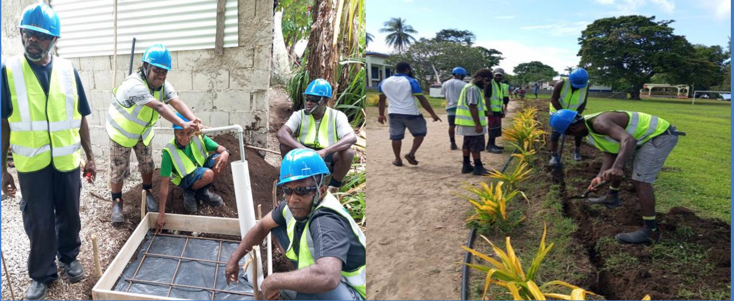
Images 3 and 4: Plumbing trainees completing a practical training component on Vao Island by aligning water pipes from a local desalination plant to a community residential area
