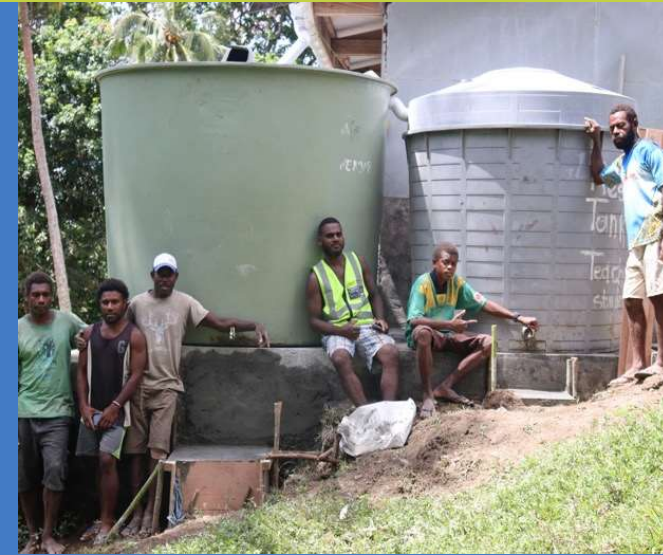
Image 2: A team comprised of volunteers from Merelava helping to build a community water system
