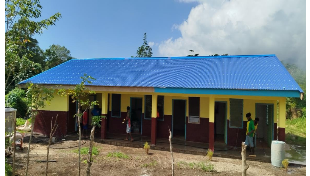
Image 6: A front view of the vanilla storage unit on Aneityum taken during a mandatory quality check of the building.
