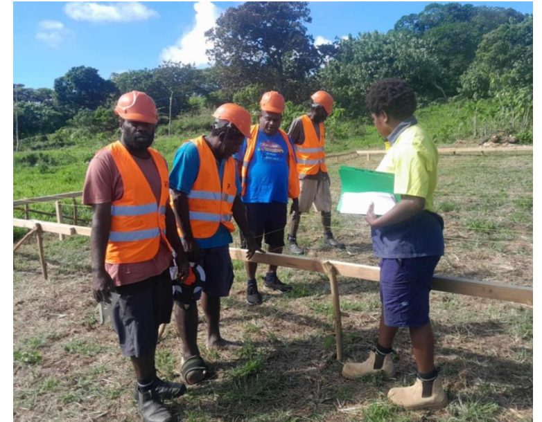
Image 6: Mary overseeing workers on site at the construction of the Central Tanna Area Council House
