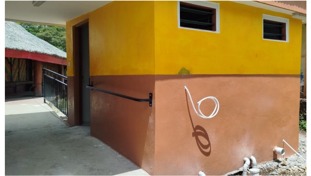
Image 10: The newly built accessible washroom facility at the National Chief's Nakamal, Port Vila.
