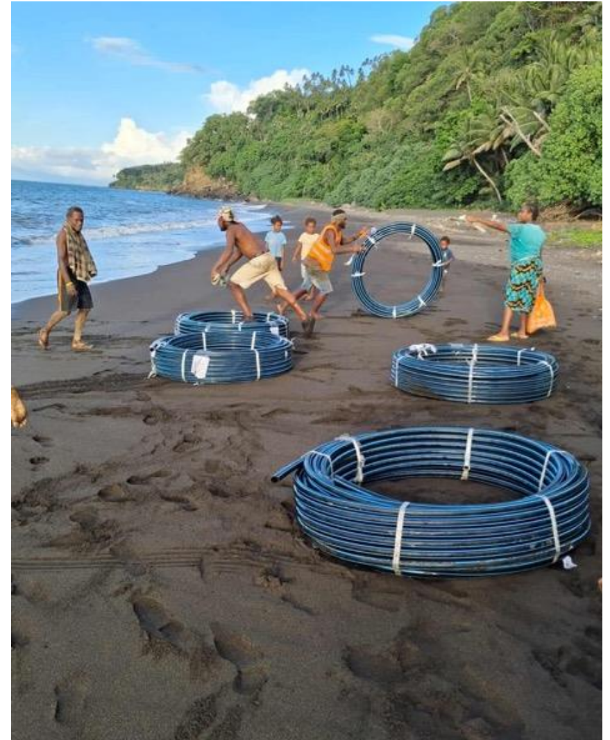
Image 3: Distribution lines for WASH systems upgrades arriving by ferry at Vandue, North Ambae.
