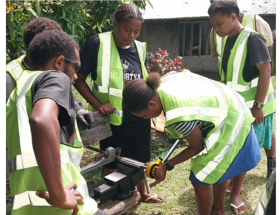
Image 8: Women involved in the village plumbing workshop and in the construction of the water supply system.
