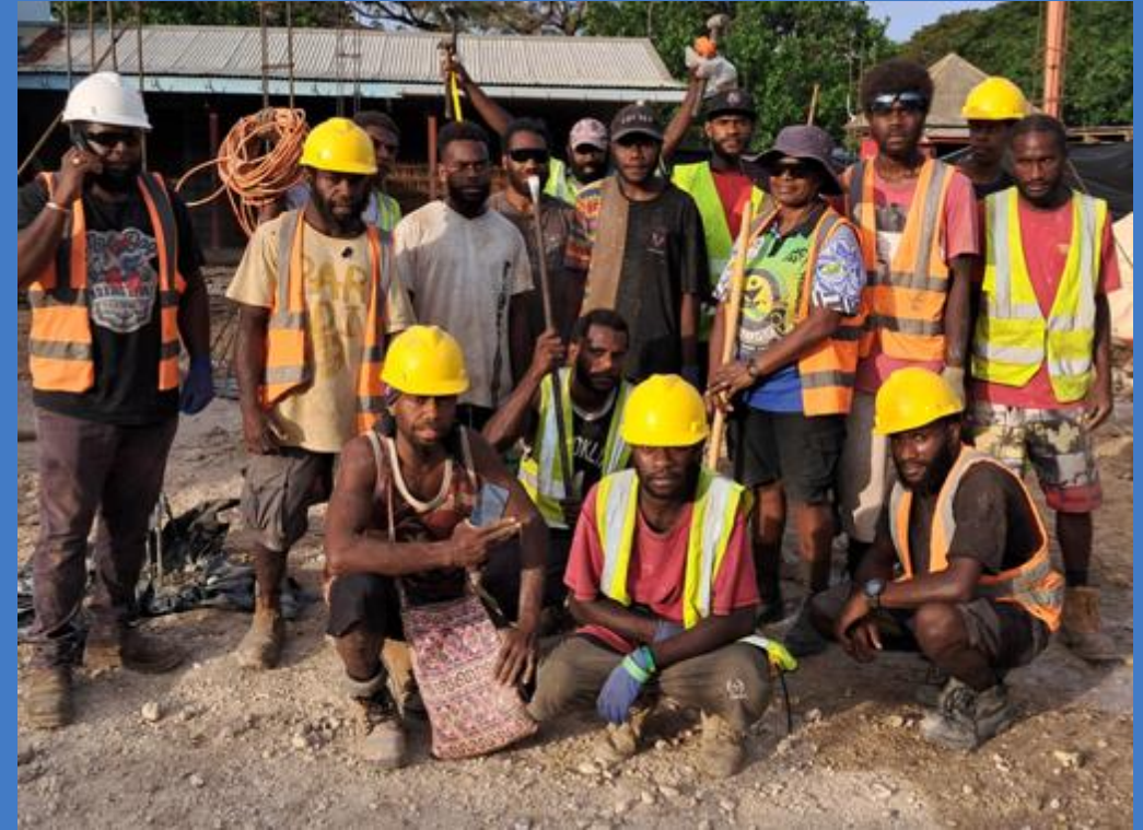
Image 18: Members of the Malekula North Central South (MNCS) Construction company posing at their work site during the construction of the new wing of the Lakatoro Market House.
