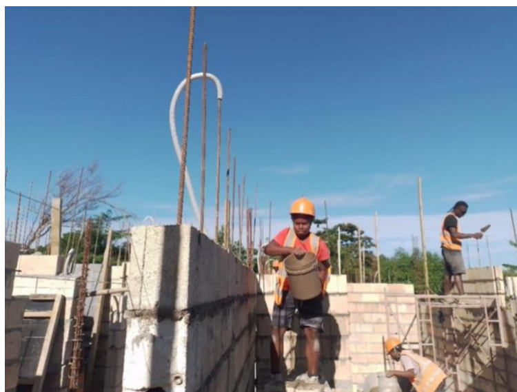
Image 8: Members of Nojavan Construction on site during the construction of the Tasmate Health Centre, West Santo
