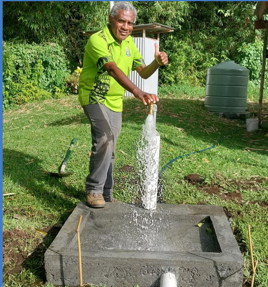
Image 1: Community leader with a tap stand connected to the new water system at Lolopuepue in North Ambae.
