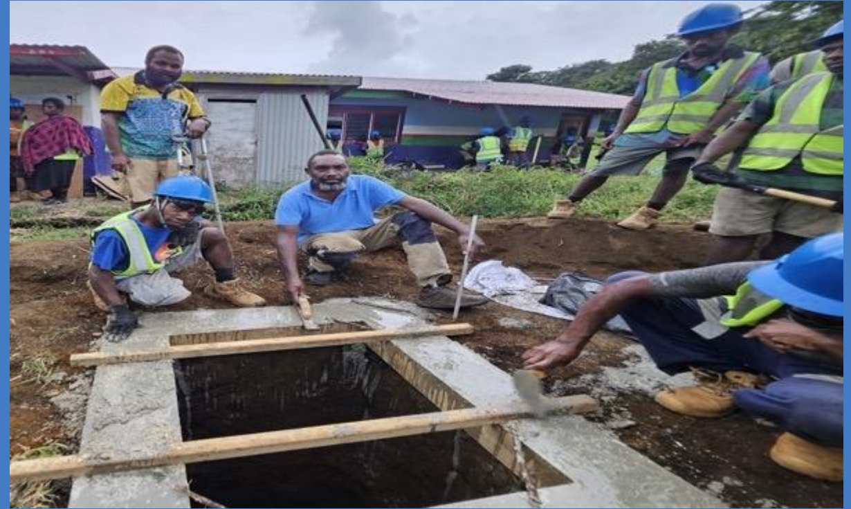
Image 11: Disability Desk Officer Mr. Maxwell Nasak stands with two trainees with disabilities, Mr. Ben and Mr. Edwin, during their plumbing practical—constructing a VIP toilet slab.
