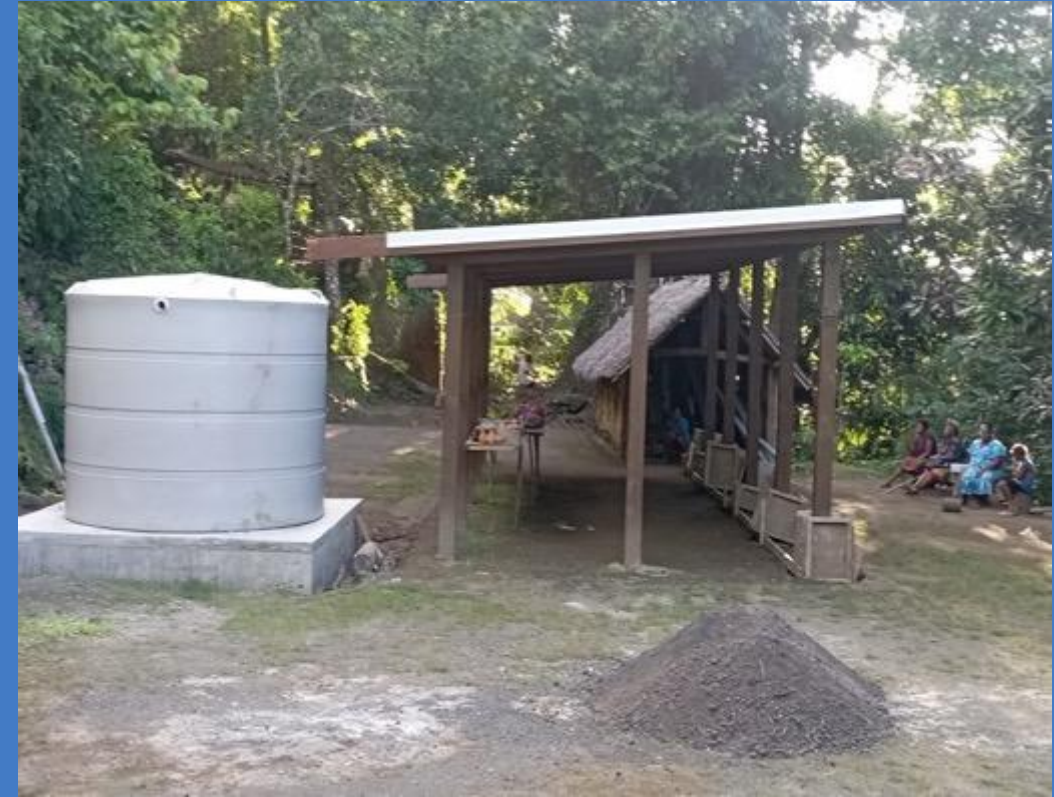
Image 2: One of the 10 rainwater harvesting systems constructed on Merelava
